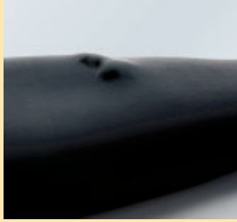
Chemical Attack: This photo shows swelling caused by oils and petroleum compounds.
